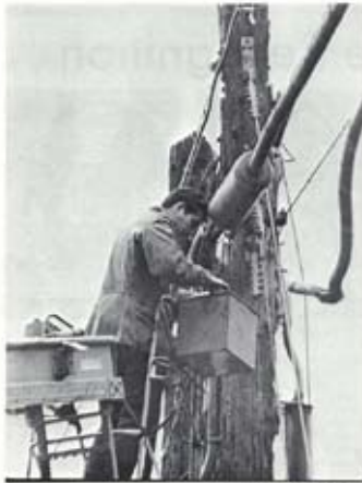
CLUE SEARCH—Centre Costa County criminologist John Murdock examines a pole damaged by blasts shortly after dawn. All three cables on the pole were damaged. After authorities finished their inspection, telephone crews were allowed to begin restoration. (More photos on page 3.)
